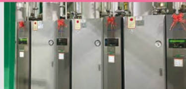
Once-through Boiler (Indonesia) DIC Corporation
