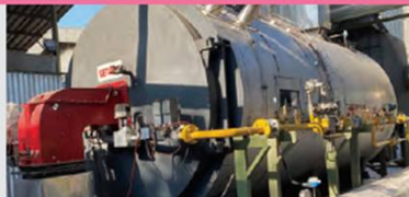
Thermal Oil Heater System (Indonesia) Fumakilla Limited
