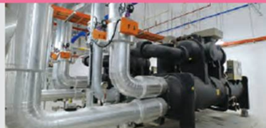
Chiller & LED Lighting (Vietnam) Tokyu Corporation
